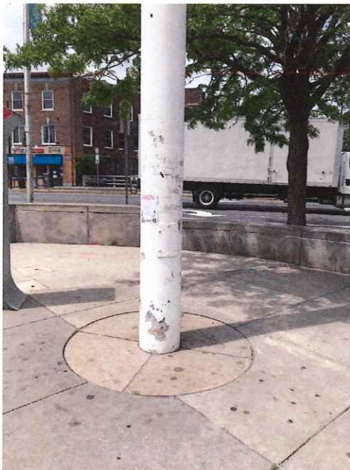
Left: flaking paint at bottom of the pole. The station contractor originally applied the pole's paint, and it appears to be missing a zinc-rich primer layer on top of the galvanized steel.
