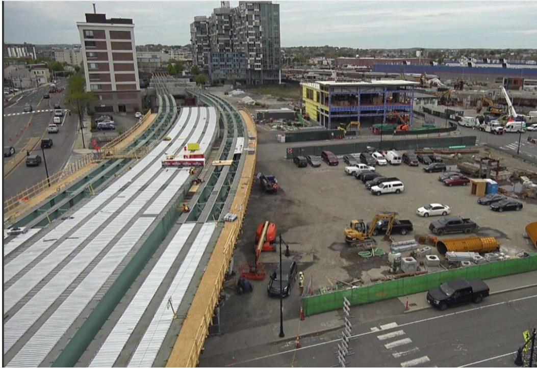
Photograph 1-View of the new Lechmere Station viaduct and platform under construction (photo courtesy MassDOT)
